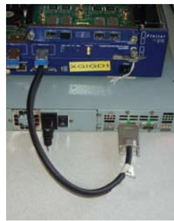
Figure 5: Appropriate Test Setup: 1) Signals are sent over a single cable, 2) the cable is a minimum length (short), and 3) the cable is properly shielded and rated for 6 Gb/s use.
